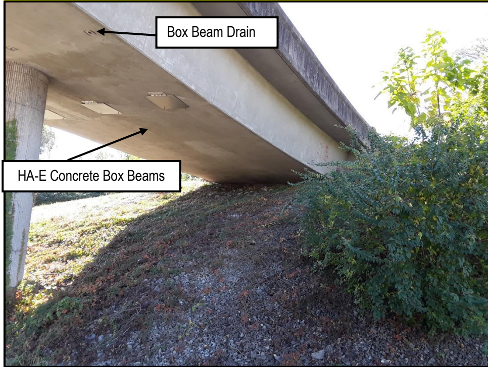
Photo 5: View of HA-E and box beam drain on the SR-1 Ramp over I-440
